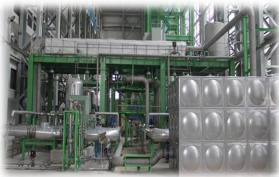
Integral Scale Hydraulic Test Facility, ISHY
